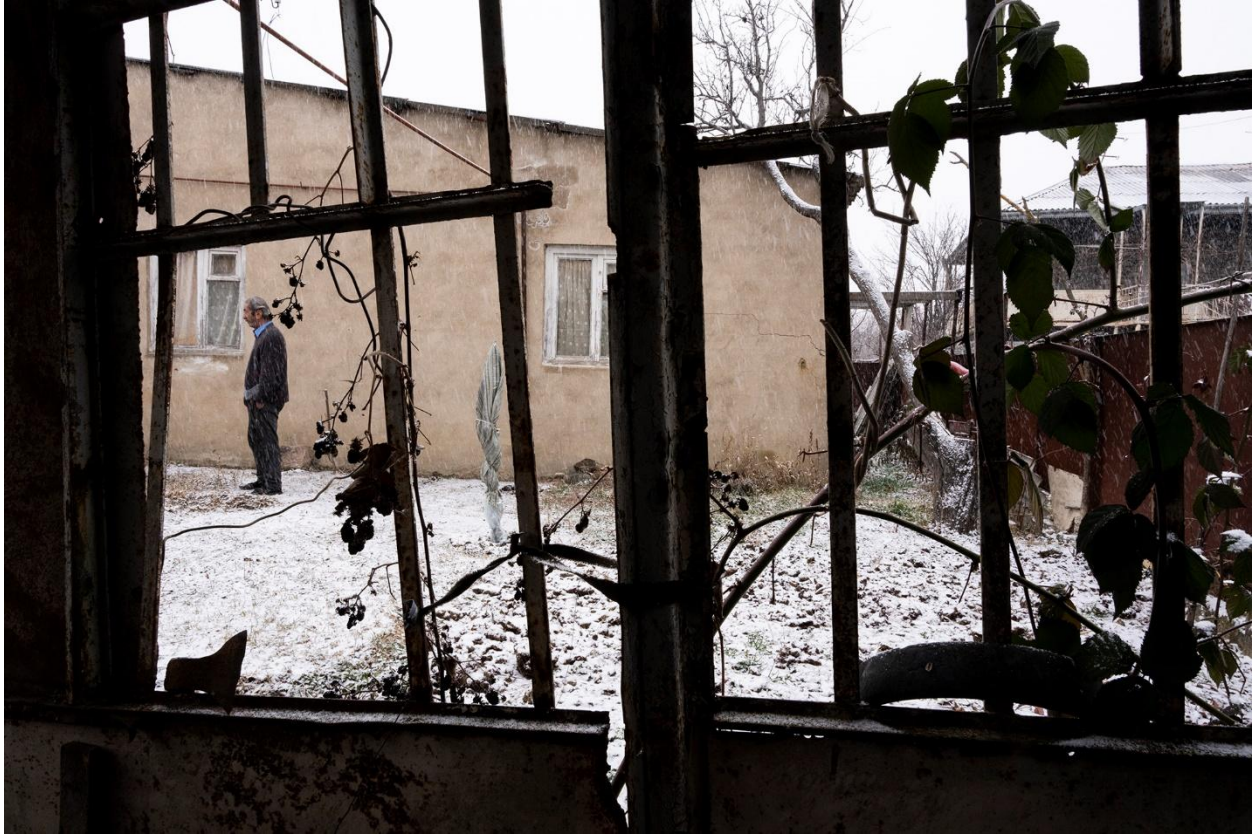
Resident of Zaardiantkari stands in front of his damaged home. Foto: Tamta Gokadze, Zaardiantkari on 15. January 2022.
